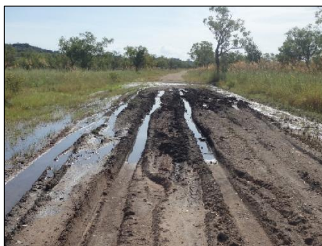
Damage to surface on closed road
