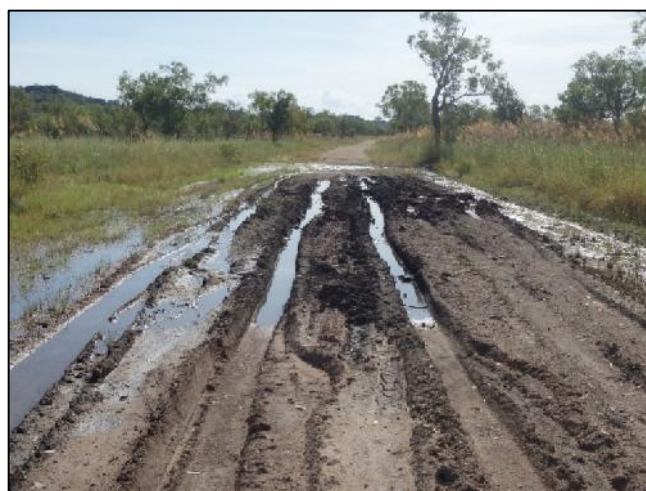
Damage to surface on closed road
